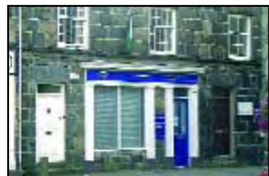
Shutters located behind glazing do not compromise the shopfront; internally lit displays can be seen through open or pierced grilles, promoting out-of-hours window shopping
