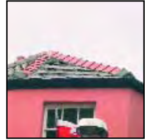
Effective repairs need to be followed through with suitable detailing – the graceful roof form and good re-slating has been spoilt by chunky hip tiles
