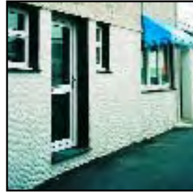
'Modernisation' of an older property using components, detailing and finishes with no local or historic relevance totally alters its character
