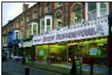
Shopfronts extending over multiple units without intermediate support, or appearing to have insufficient structure to carry upper floors, give a feeling of instability, and relate poorly to the original plot widths
