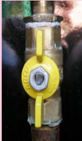
Emergency Control Valve
