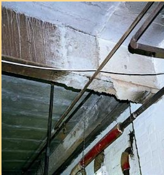
Sprayed Asbestos and Lagging.
