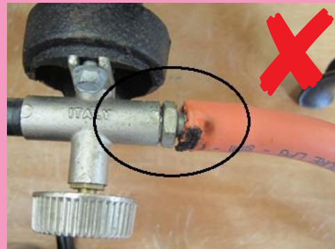
The flexible hose connection to the double ring burner has no jubilee clip. The gas reacted with the heat from the flame and caused the flexible hose to burn.
